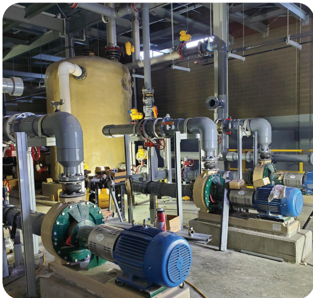
High and Low pH Cleaning Pumps and Piping Installation in the Membrane Filtration Building (02/28/2024)
