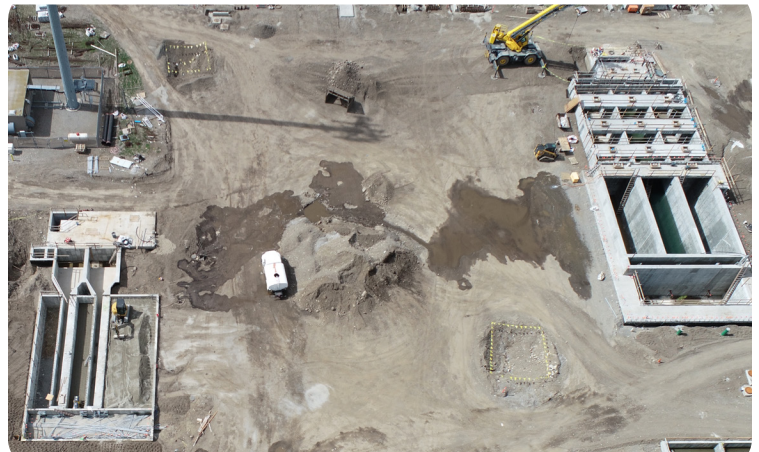
Ultraviolet Disinfection and Tertiary Plate Settler (4/1/22)
