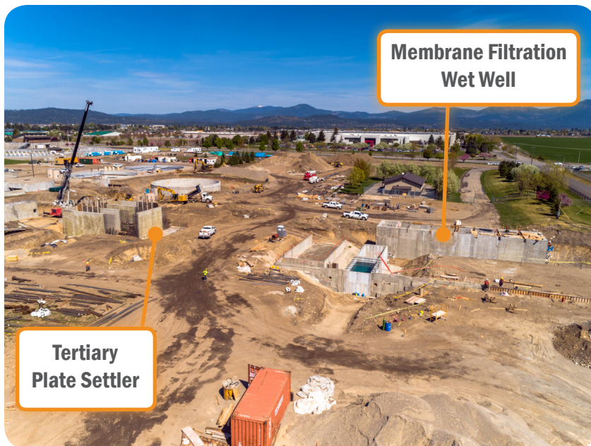
Membrane Filtration Building and Tertiary Plate Settler (5/6/21)
