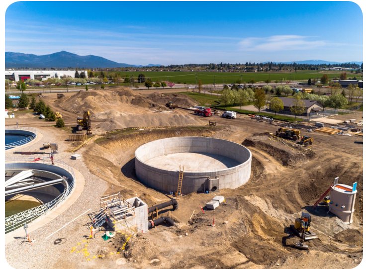
Secondary Clarifier No. 8 and Splitter Box No. 3 (5/6/21)
