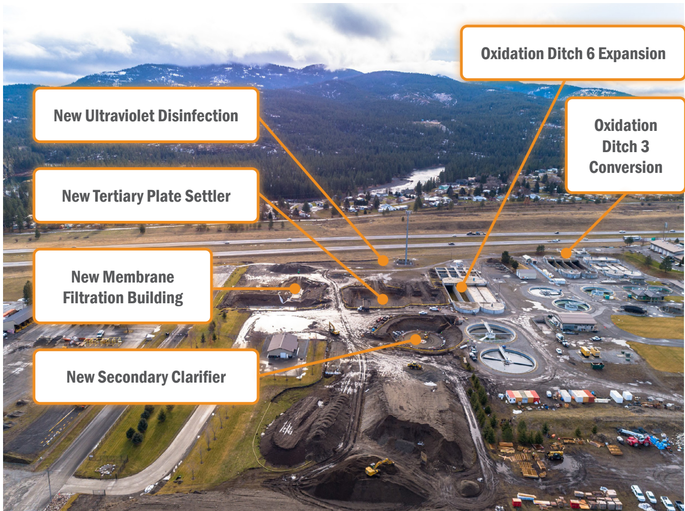
WRF Tertiary Treatment Improvements expansion area (looking south to the Spokane River and Interstate 90) (1/5/21)
