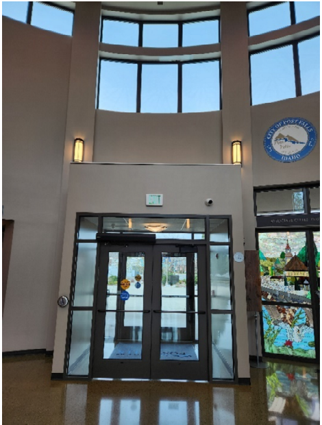
Photo #3: Rotunda drywall damage location.
