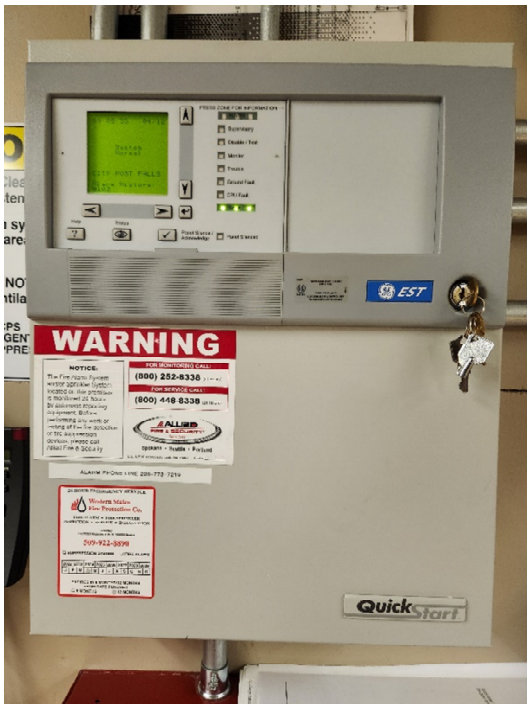
Photo #7: Fire Alarm.
