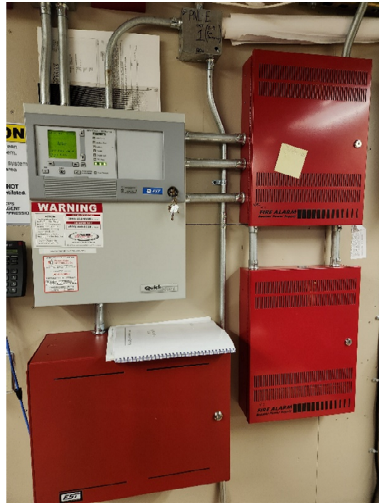
Photo #8: Fire Alarm.
