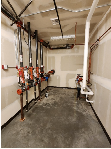
Photo #5: Fire Riser Room.
