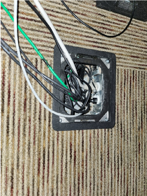
Photo #2: Council Chambers floor box.
