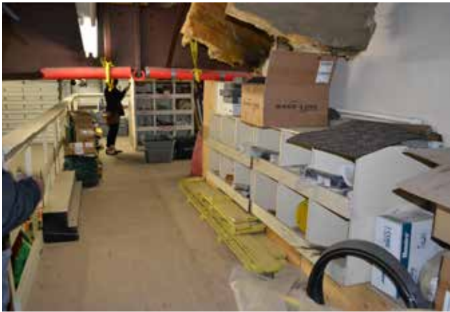
FIGURE 61. SHOP CEILING IN NEED OF REPAIR
