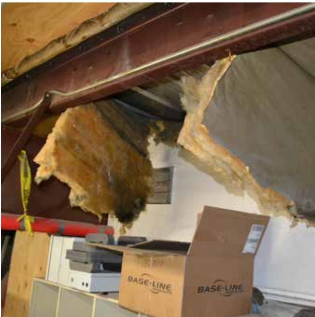
FIGURE 102. EXPOSED INSULATION AT THE PARKS M&O SHOP
