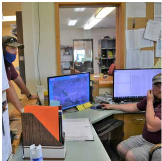
FIGURE 50. UNDERSIZED WRF SCADA CONTROL
