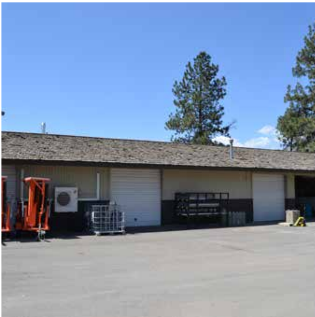
FIGURE 101. STREETS SIGN SHOP ROOF IN NEED OF REPAIR
