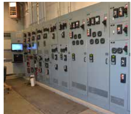
FIGURE 40. CRITICAL ELECTRIC PANEL IN UTILITY BUILDING 2
