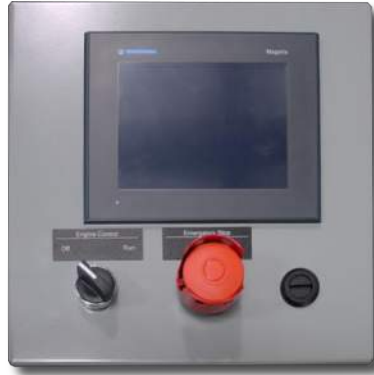
Figure 5: Remote Engine Control Panel
