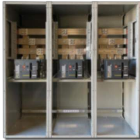
Figure 2: 500kW, 480V, 800A Paralleled Generators Disconnect & Output Protection Insulated Case Circuit Breakers and load take-off
