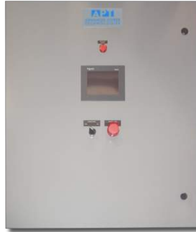
Figure 8: Remote Generator Start/Stop & Setpoints Panel
